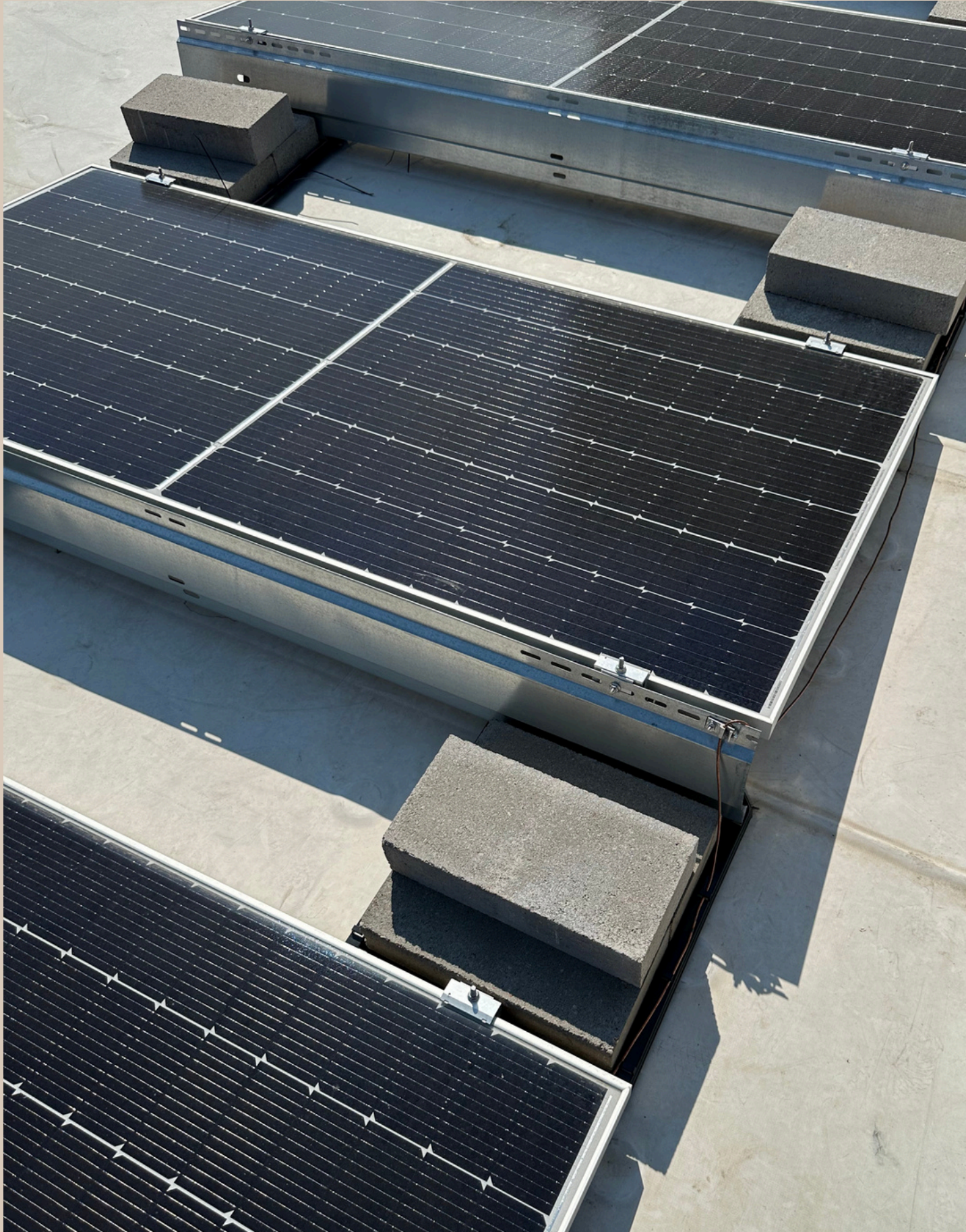
Solar panels at Backyard on Blake
